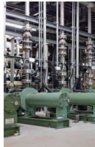
超純水製程高壓泵 Oil Pump Cooling System
