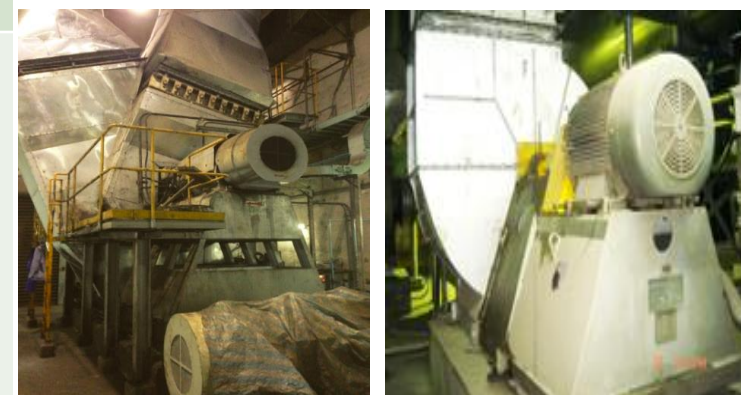
▲ 焚化爐誘引抽風機550KW
